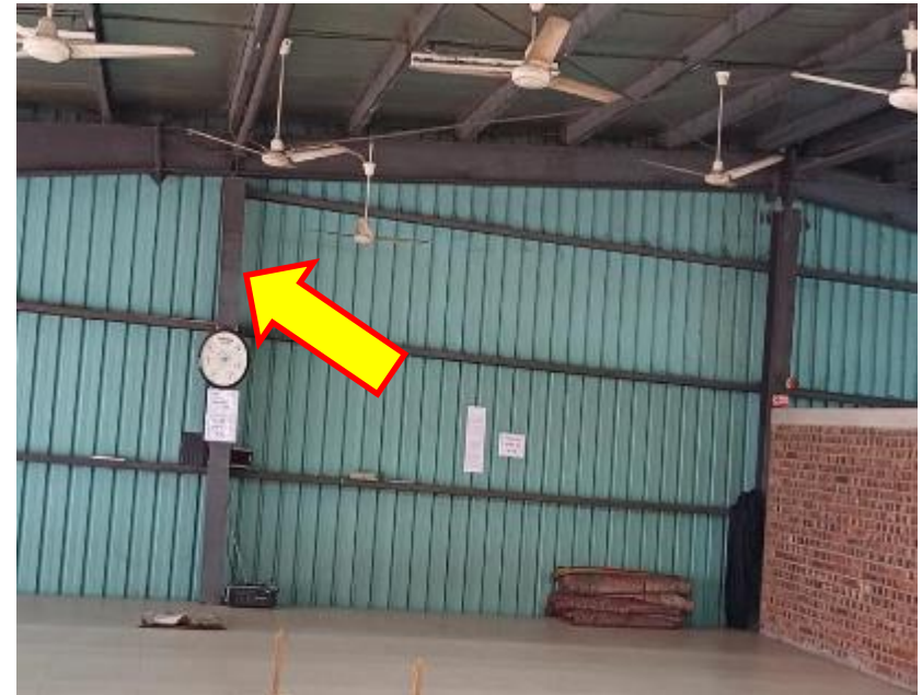
Rotated column above floor
