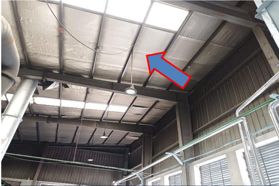
Compression member, wall & roof bracing missing
