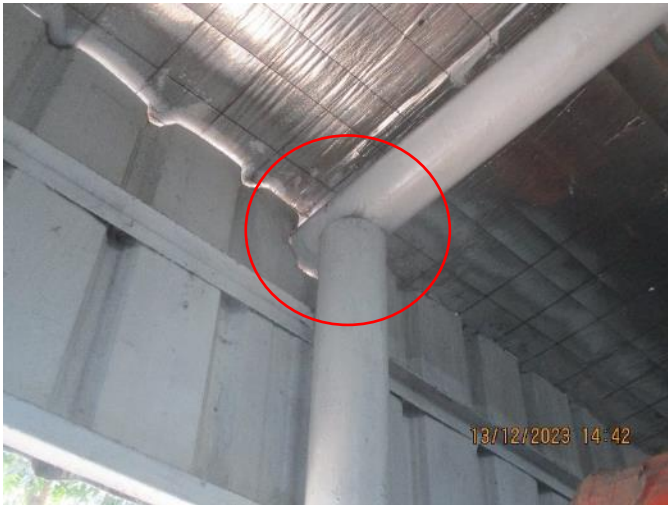
WP maintenance workshop shed
