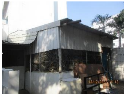
WP maintenance workshop shed
