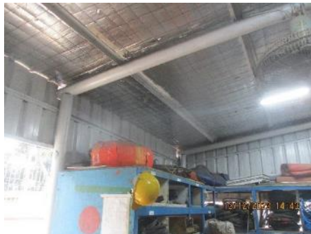
WP maintenance workshop shed
