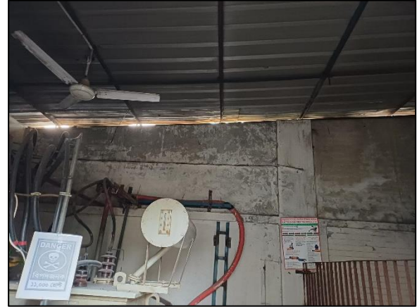
Shed 5-Substation Shed
