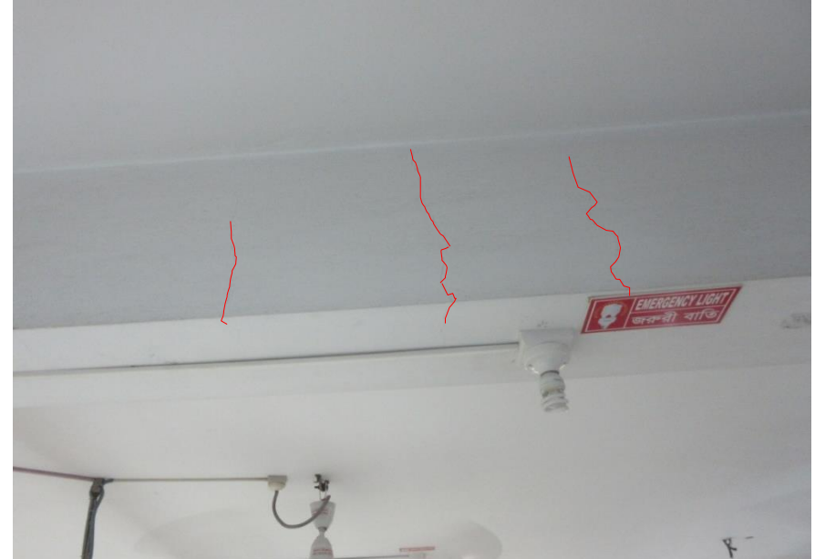
Cracks observed at almost all beams.
