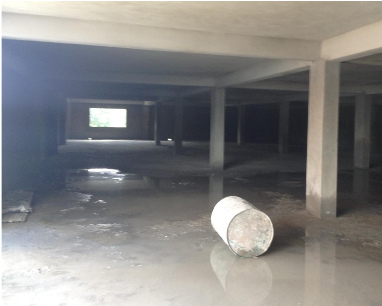
Standing water observed on 1st floor slab
