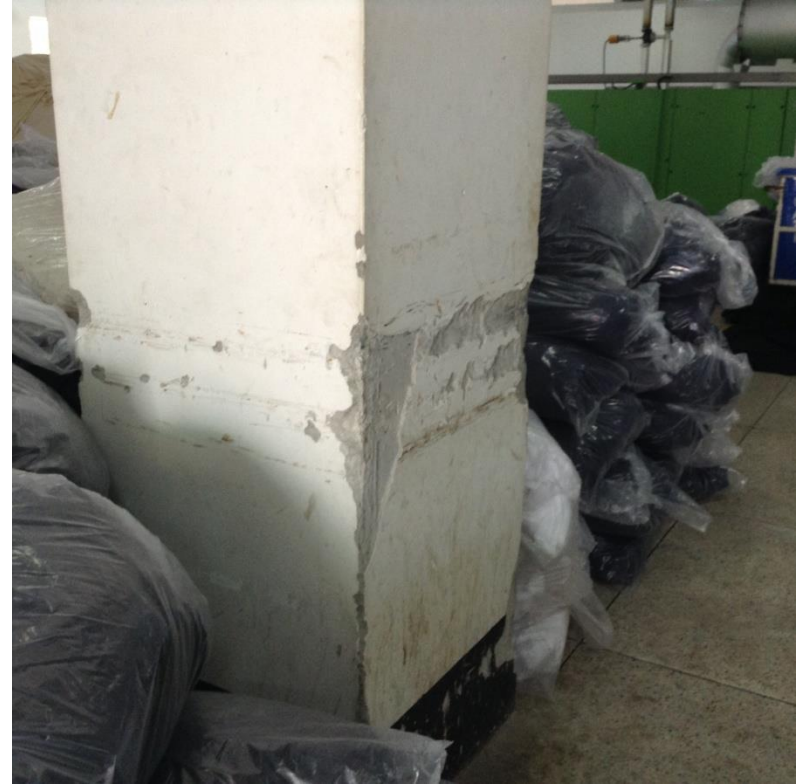
No Protection around column area at ground level.
