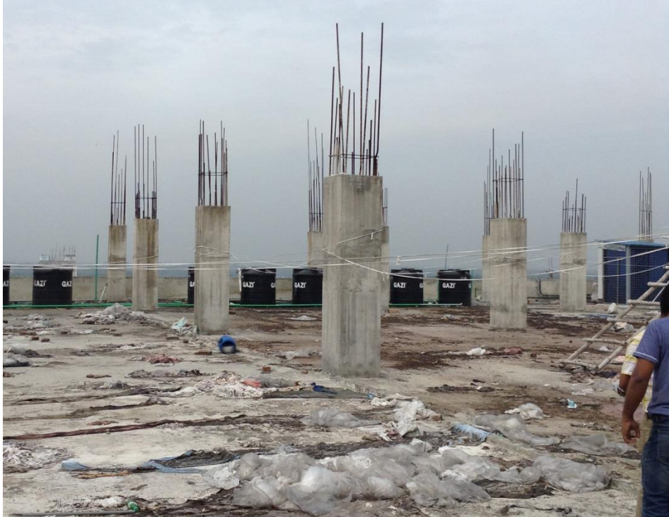
Steel Bars were exposed from the roof column and corrosion may take place in near future.
