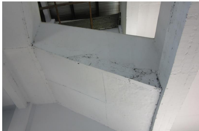
Insufficiently compacted concrete
