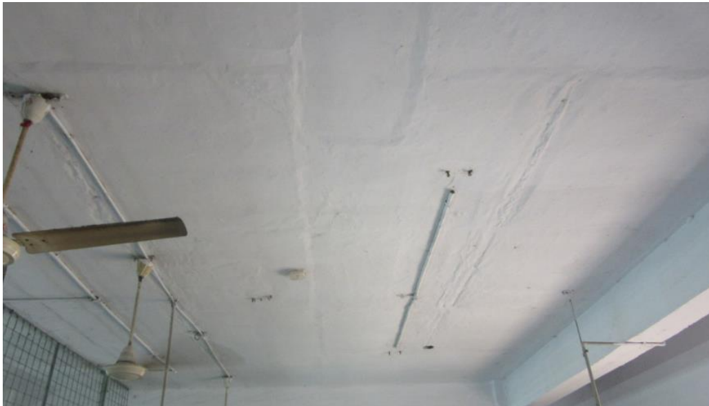
Uneven slab due to bad formwork
