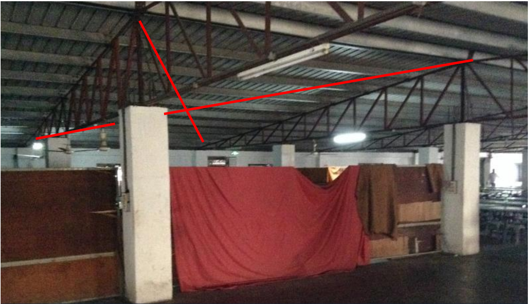
Lack of bracing in roof structure
