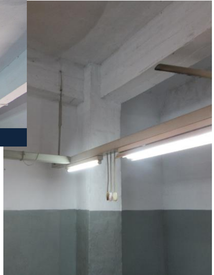
Uneven slab due to bad formwork
