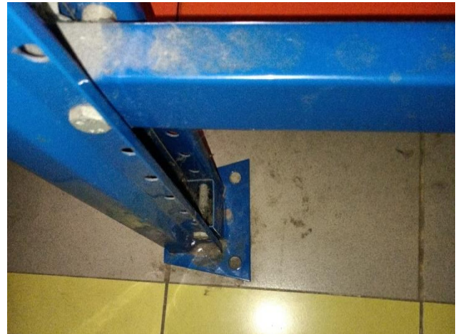
Unbraced racks on floor
