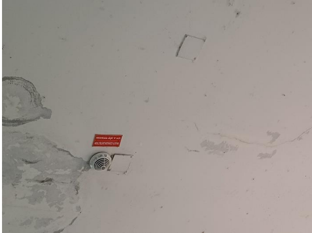
Cracks on slab soffit
