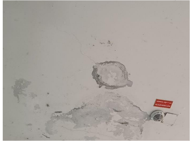
Cracks on slab soffit
