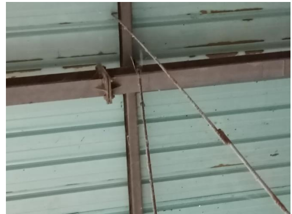
Gap between endplates of steel rafter
