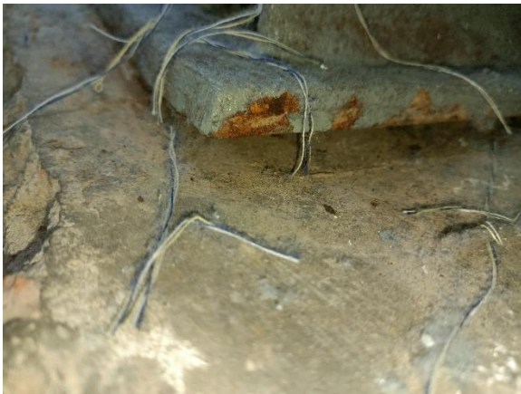
Gap between baseplate and pedestal column
