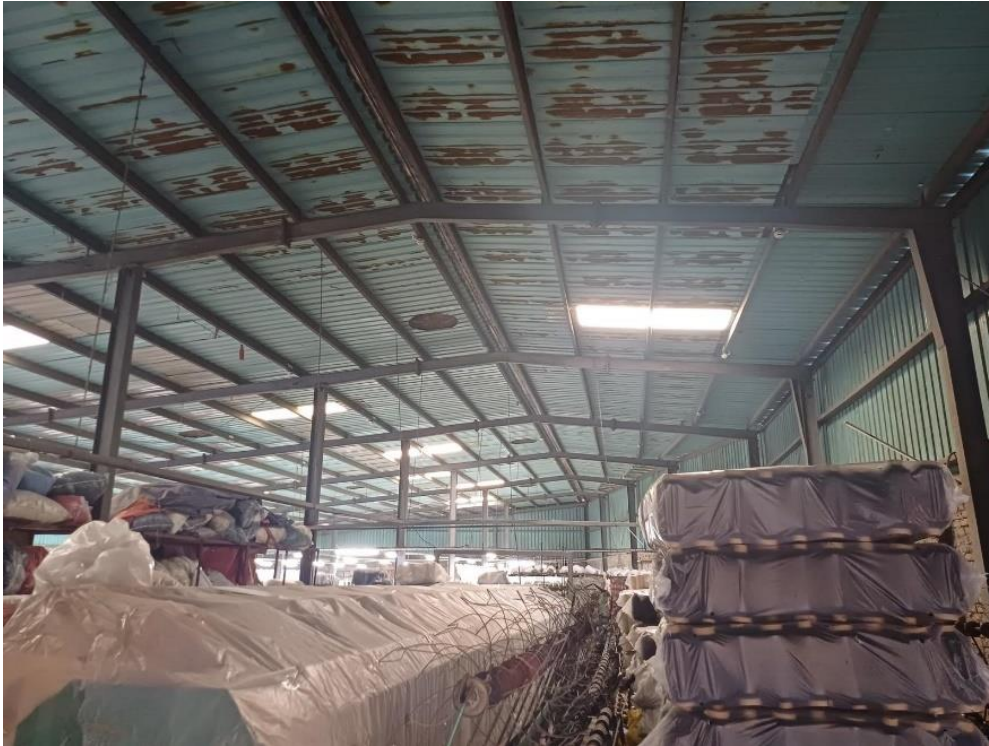
Absence of load transfer media (Compression Strut) along transverse direction of rafter
