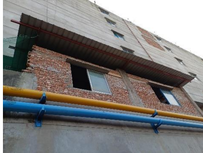
Filter Press M/C Room
