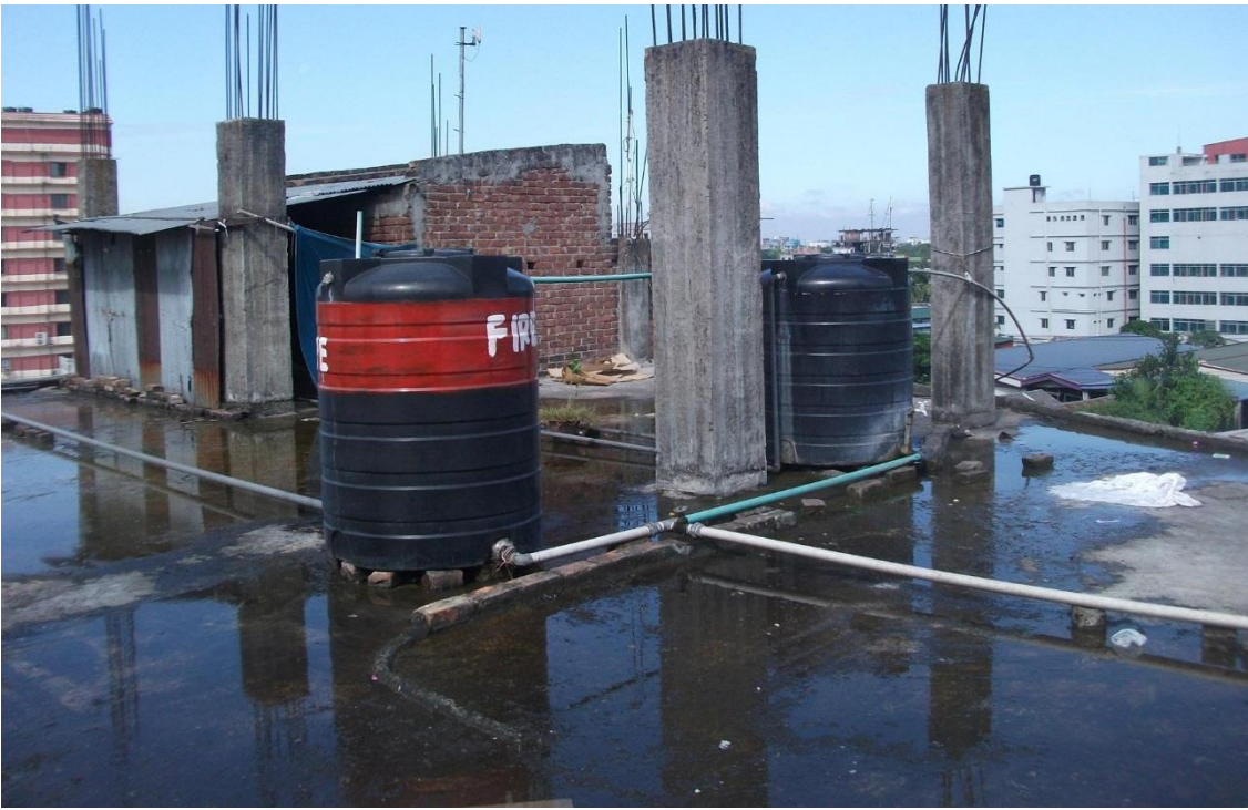
Significant water accumulation observed at roof level.
