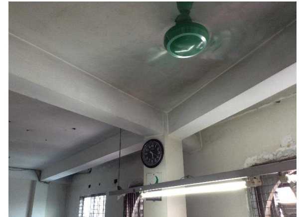
Moisture was observed due to water ingress at 3rd floor under Roof slab causing deterioration of structure
