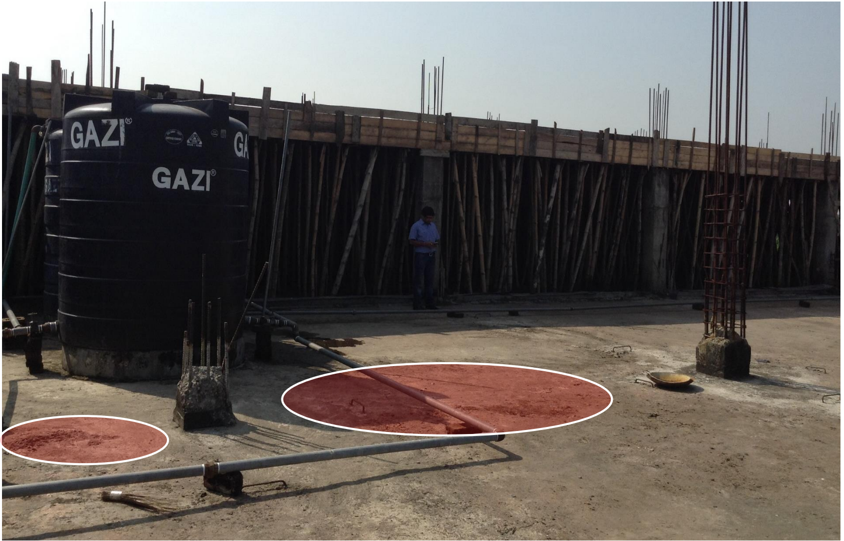
Water Ponding on Roof Causes Dampness on Slab Soffit Below
