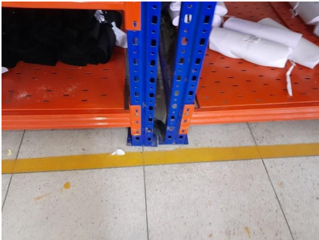
Storage Rack – not anchored
