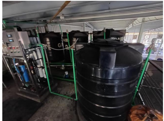
Plastic Water Tank on mezzanine roof not braced
