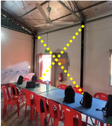
Bracing Missing in side wall
