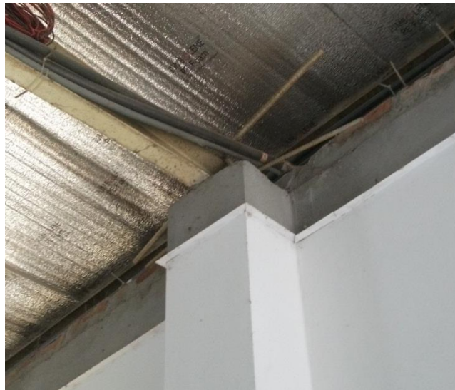
Steel truss resting on top of the RC column at edge. Proper connection was not observed. Exposed rebars are tied and welded to steel profiles.
