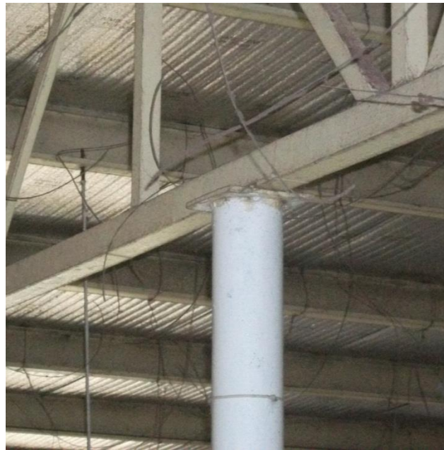
Poor welding between Steel Post to Truss bottom flange
