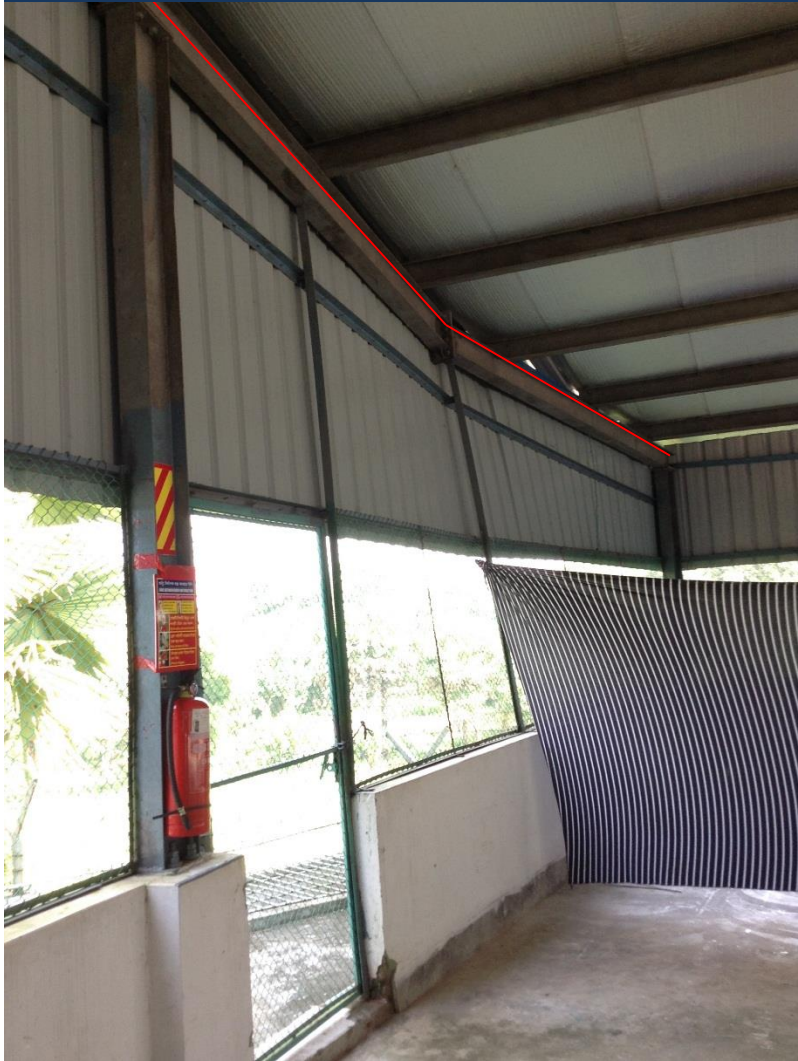
Lateral buckling at mid rafter
