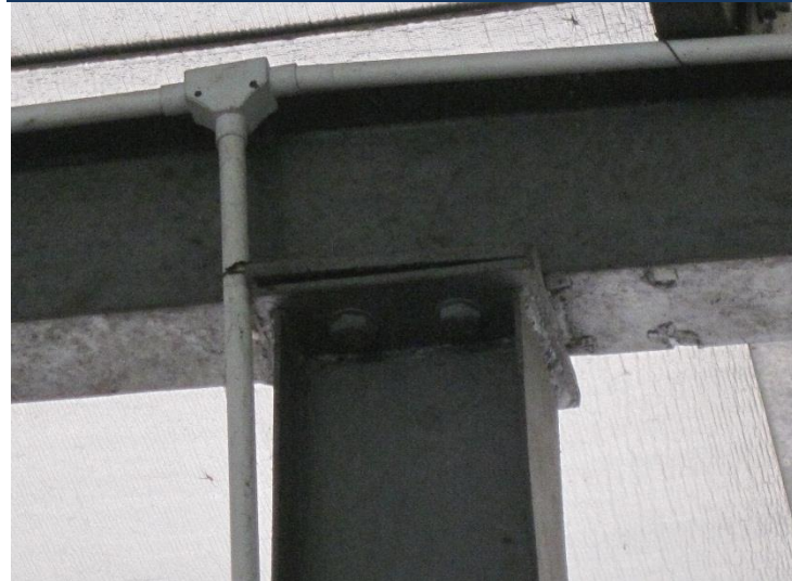
Gaps in bolted connections
