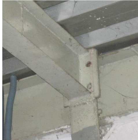
Missing bolts under mezzanine floor of main factory (finished good ceiling)
