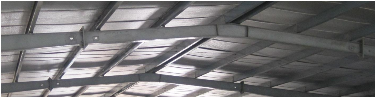
Lack of lateral braces in warehouse roof
