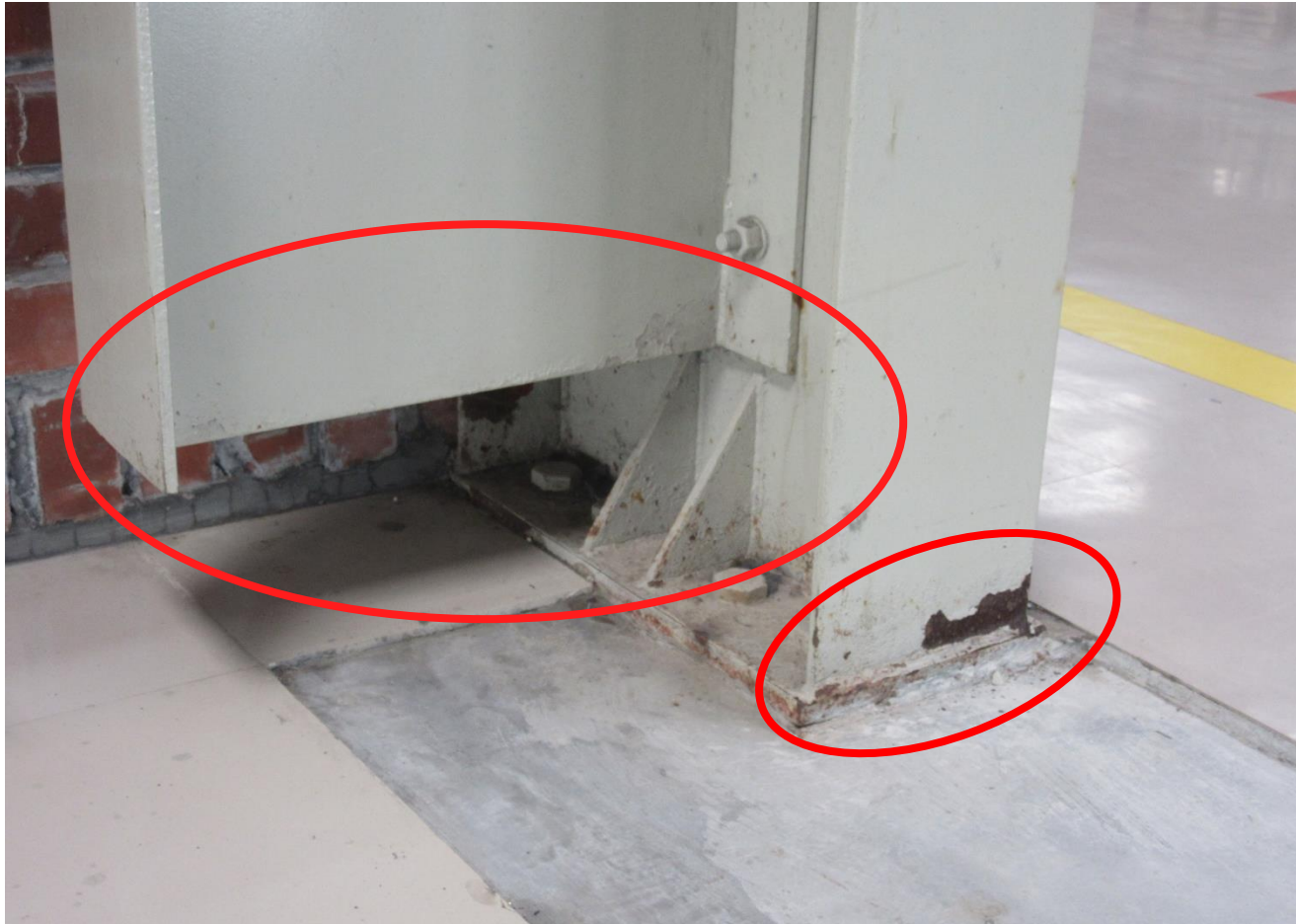
Discontinuity and Corrosion found in the portal frame bracing at column F-17
