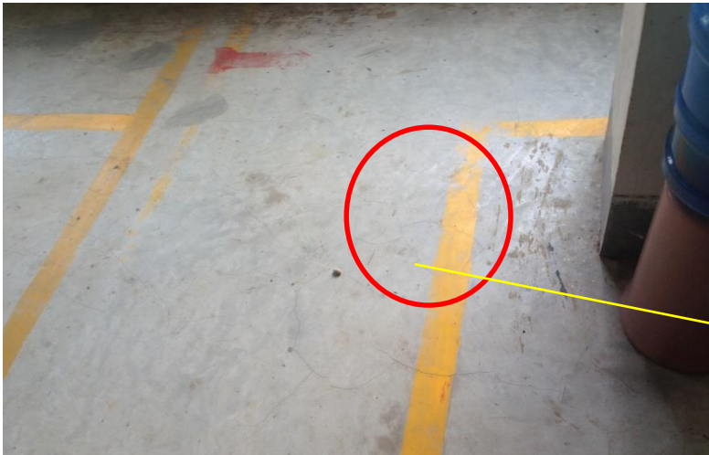
Observed cracks in floor slabs in Building 2
