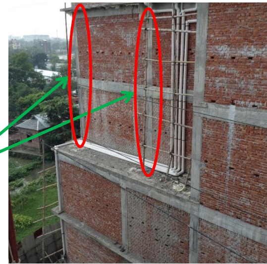
Observed columns which are shifted inwards after the 2 nd floor.
