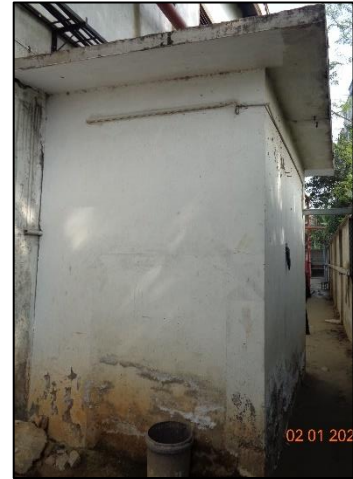
Sludge storage room (dampness on wall)
