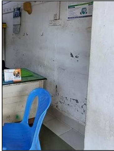
Guard Room (dampness on wall)
