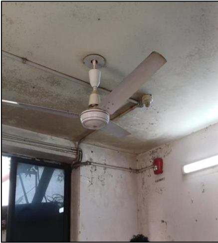
Access control room (dampness on slab)
