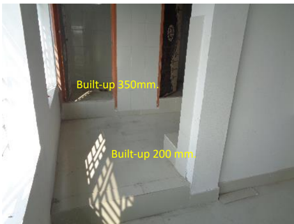
Undocumented toilet built up at second floor.
