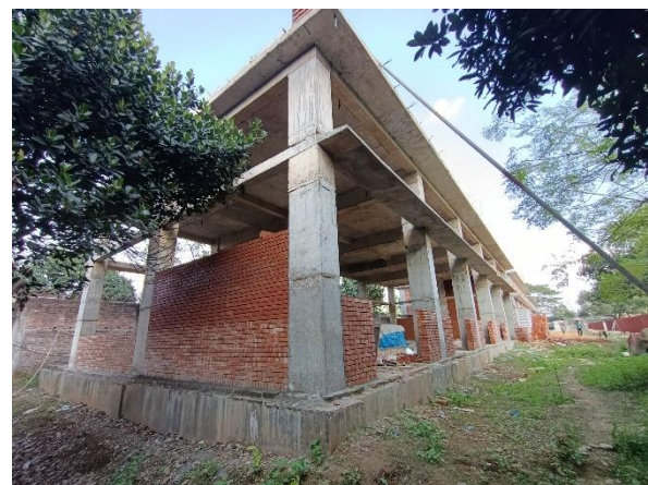
Boiler & Compressor Building
