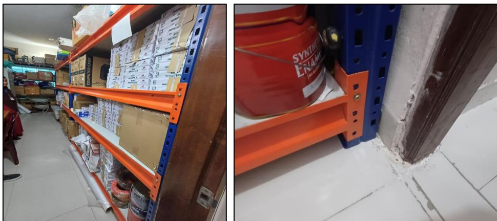
Unbraced storage racks on floors
