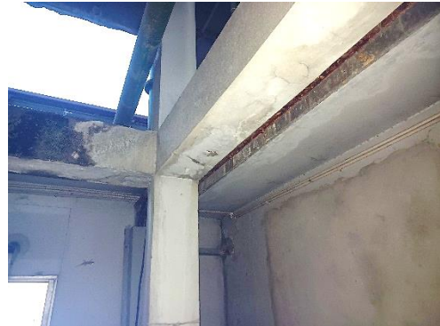
Cracks on beam
