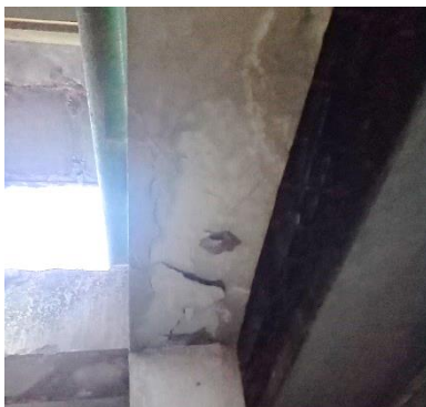
Cracks on beam
