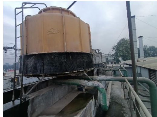
Cooling Tower (roof)
