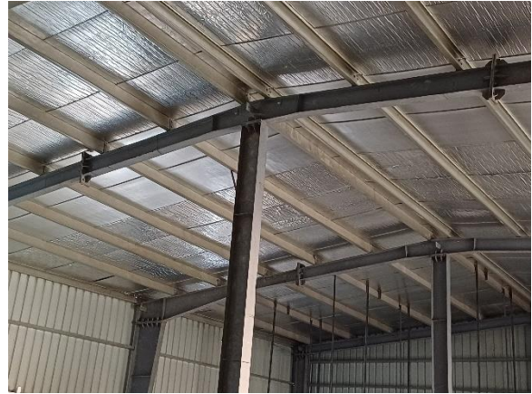
Missing compression strut
