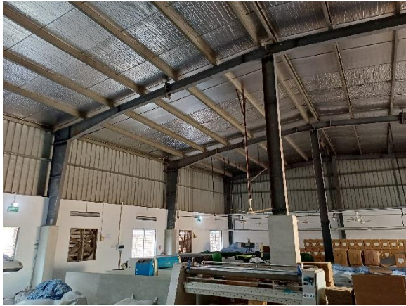
Missing wall bracing and roof bracing
