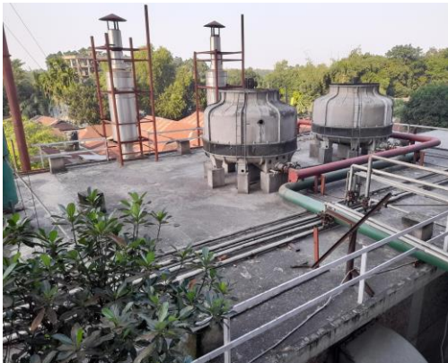
Roop top chiller
