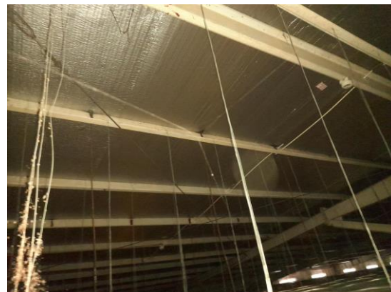
Cable bracing on roof
