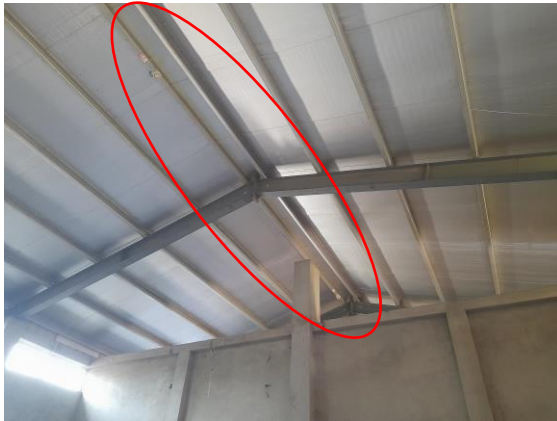
Missing compression strut
