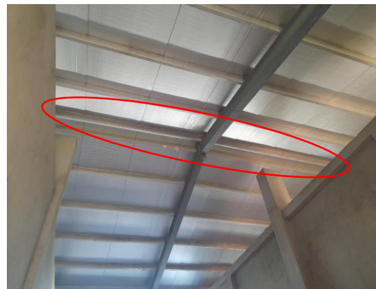
No vertical or Horizontal bracing
