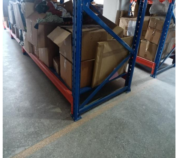
Racks without anchorage
