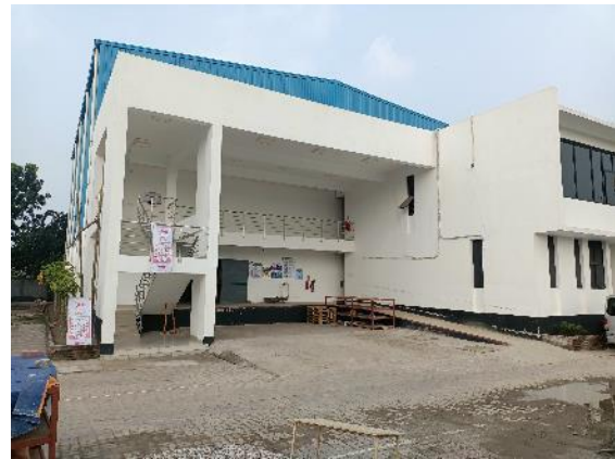
No beam at +4.8 m level
