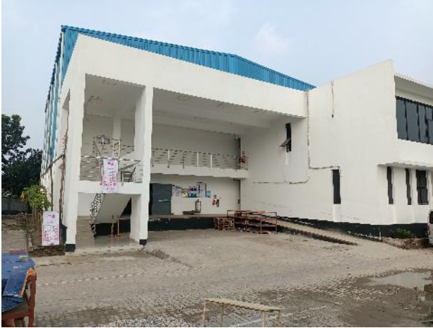
Vehicle impact risk on column
