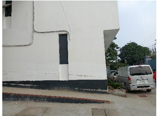
Trolley impact on column
