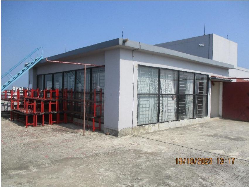
Falling hazard from stair roof top
