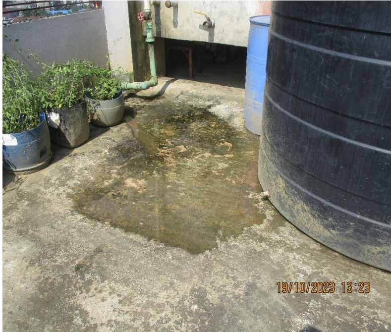
Water ponding on the roof
