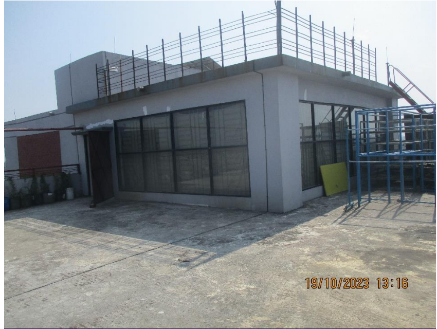
Falling hazard from stair roof top
