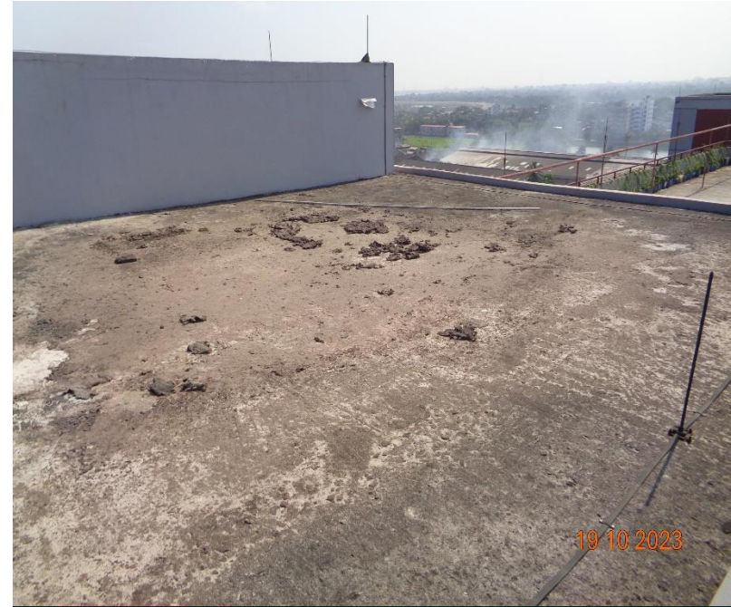
Signage of water ponding on the roof
