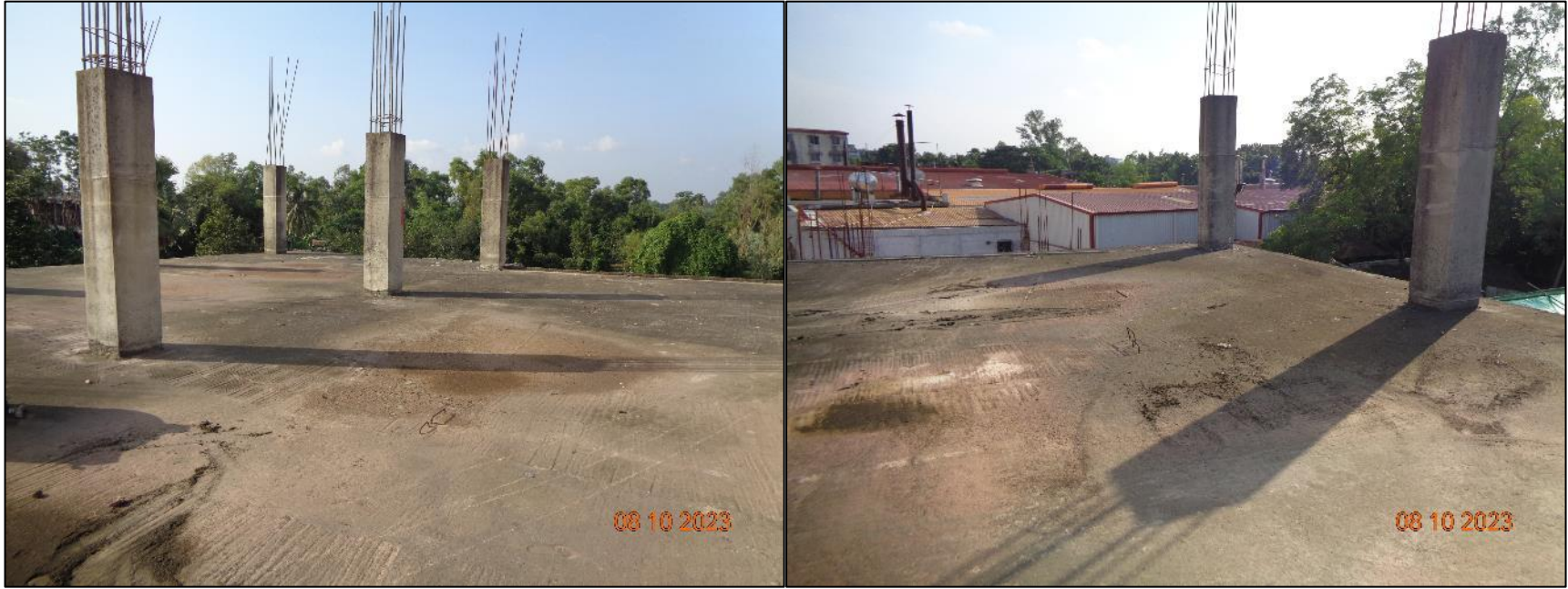
Parapet wall missing at roof
