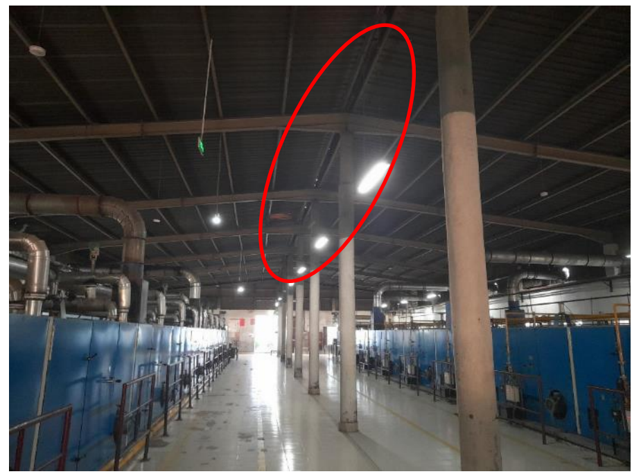
No bracing/Compression strut was provided along the long direction.
