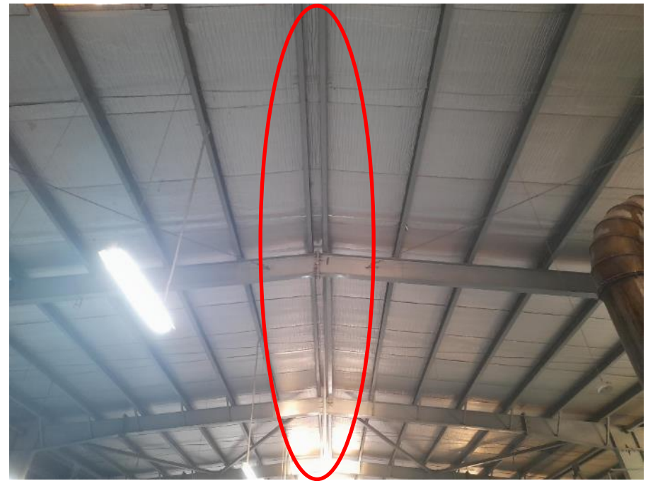
Bracing/Compression strut were missing in some grids along the long direction.
