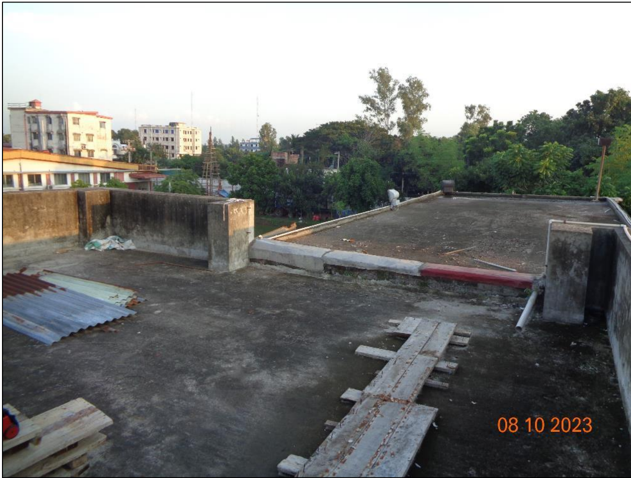
Parapet wall missing at roof
