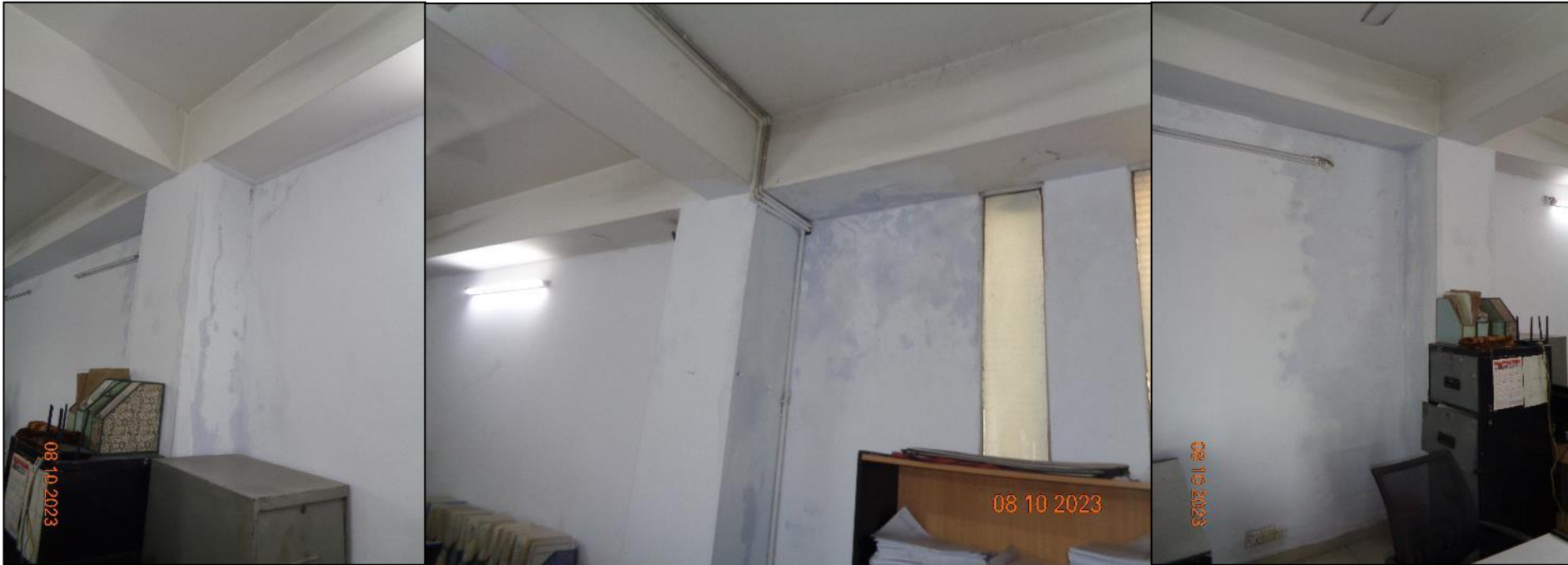
Dampness on beam, Column and wall
