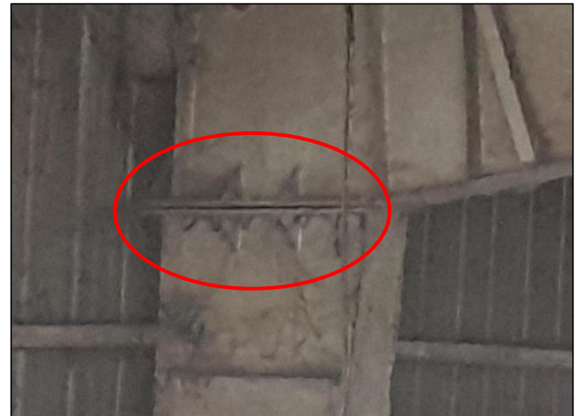
Gap observed in connections
