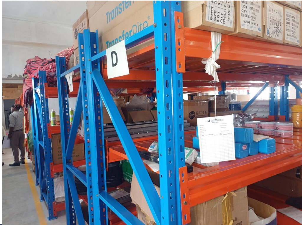
Lack of anchorage of storage rack
