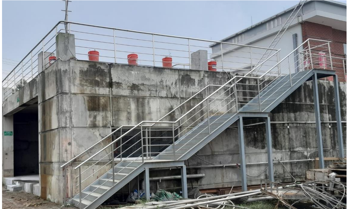
Dampness on Exterior wall
