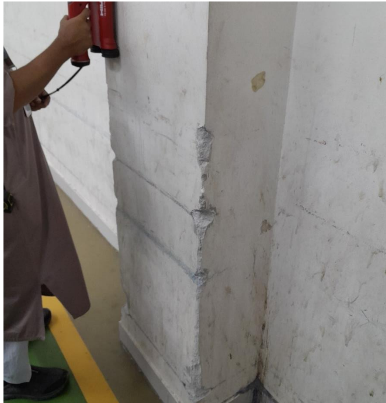
Damage RC Column due to trolley
