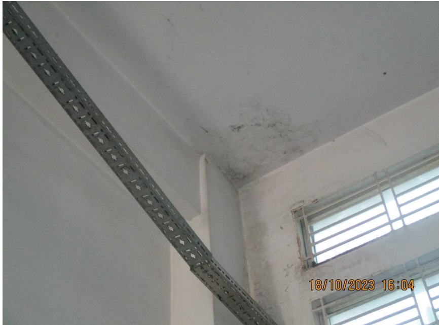
Dampness on slab soffit
