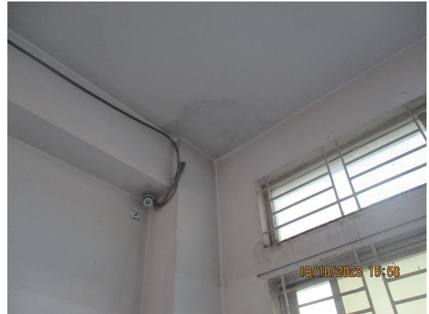
Dampness on slab soffit
