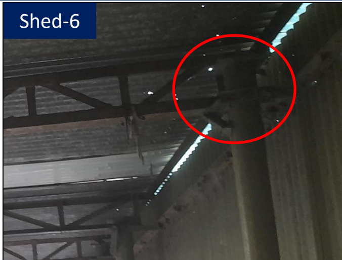
Poorly welded truss with steel pipe
