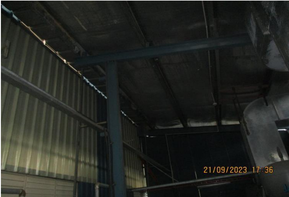
Absence of bracing system
