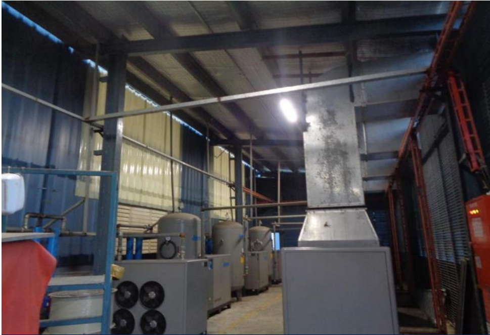
Absence of bracing system
