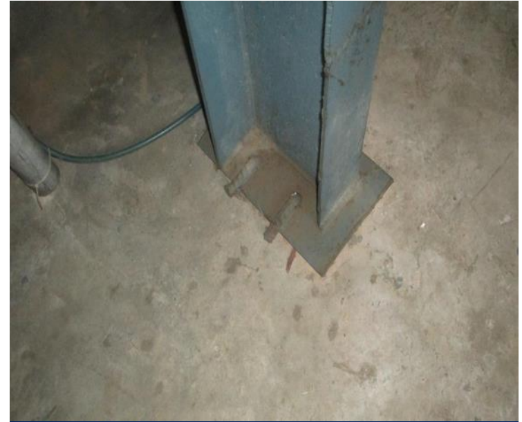
Improper connection between steel column and pedestal
