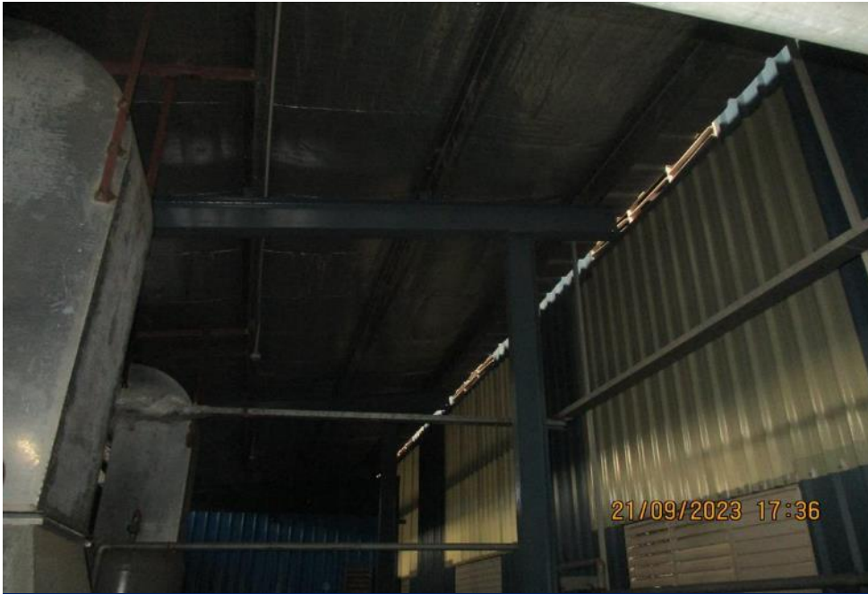
Absence of bracing system
