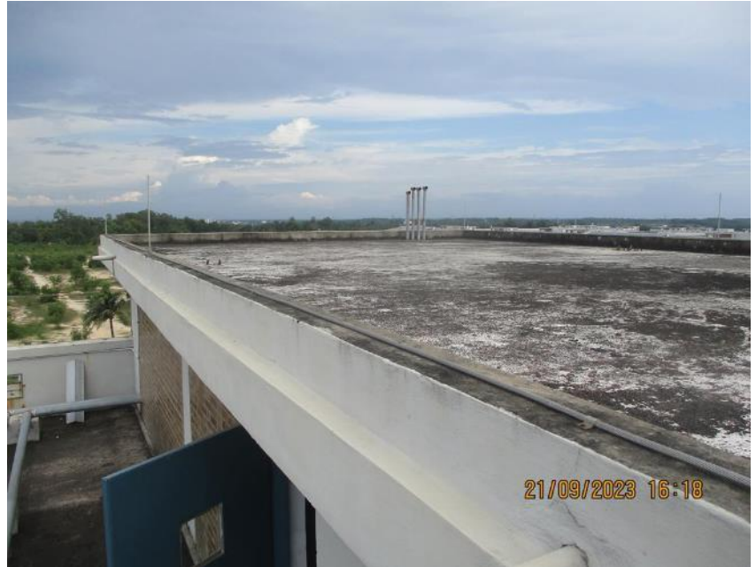
Falling hazard from stair roof top
