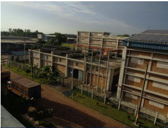
4 th phase sub-station
