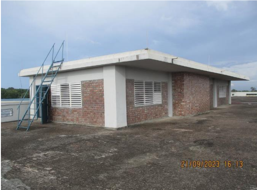
Falling hazard from stair roof top
