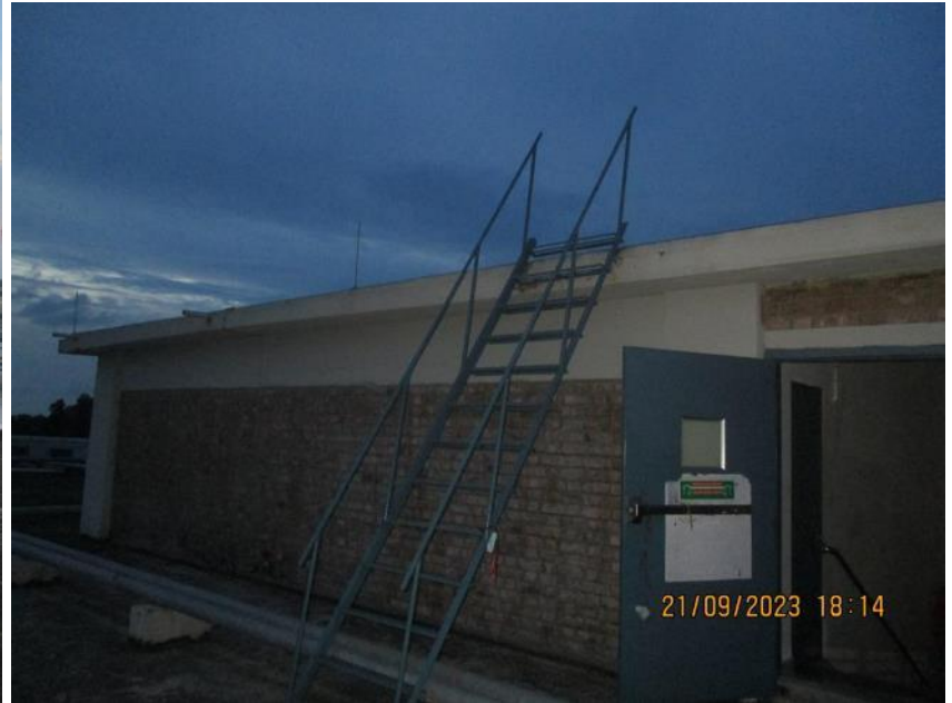
Falling hazard from stair roof top
