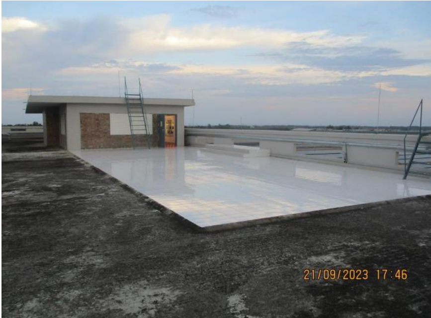
Falling hazard from stair roof top
