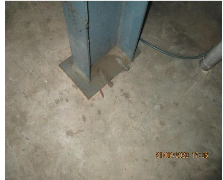
Improper connection between steel column and pedestal
