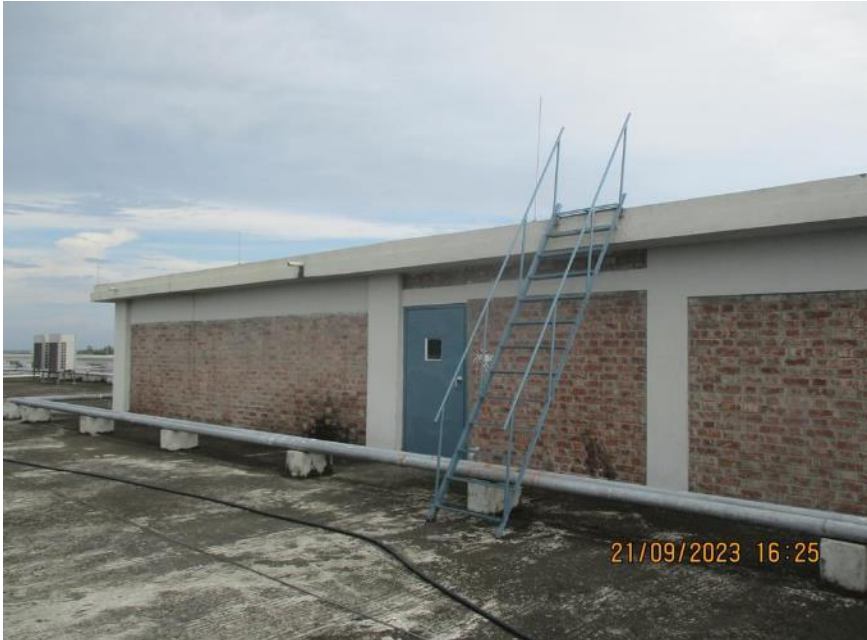
Falling hazard from stair roof top
