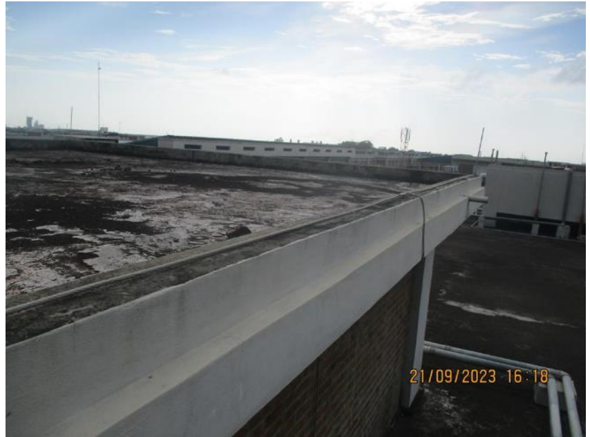
Falling hazard from stair roof top
