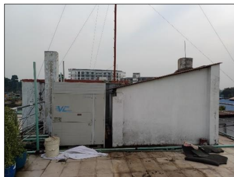
OHT, tower & electrical equipment at roof
