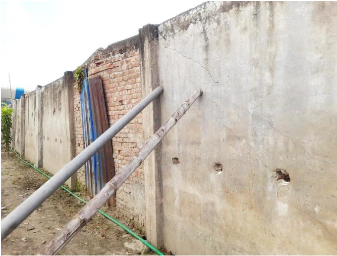
Leaned Boundary wall
