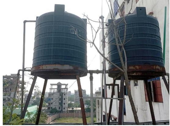
Corrosion on the water tank supporting structure
