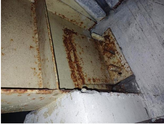
Corrosion on the steel beam
