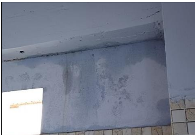
Dampness in periphery wall
