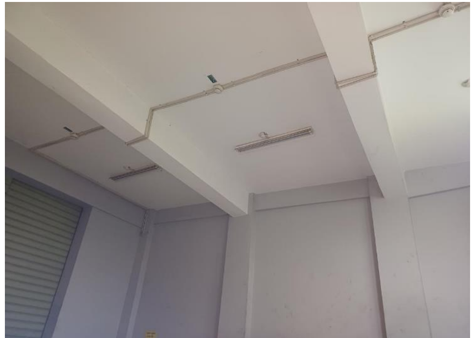
One way slab was found on-site
