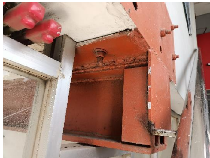
Bolt missing at connection
