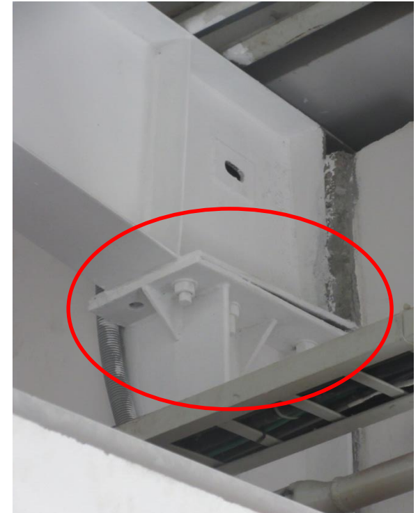
Bolt missing of connection on North side in production building also in stair side of dining building
