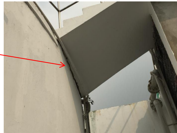
Outer side wall has water leakage
