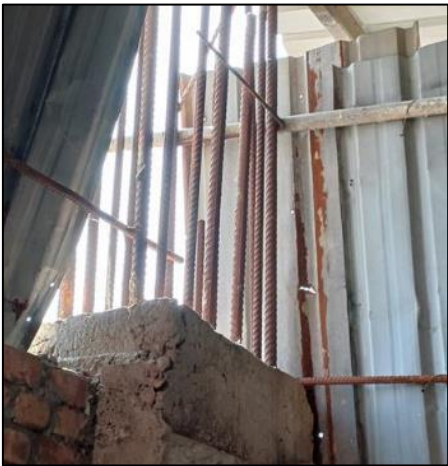
C5 column-18 nos of rebar found instead of 24 nos rebar.
