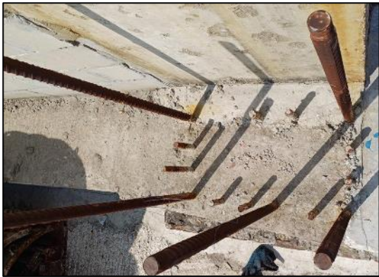
C2 column-16 nos of rebar found instead of 18 nos rebar.
