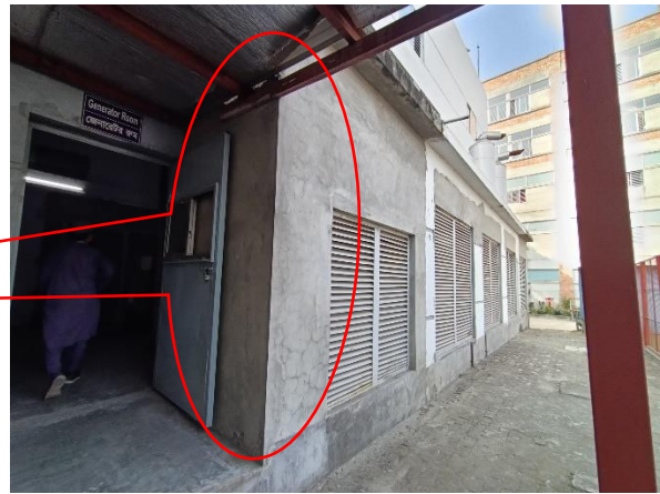
Undocumented column on GF
