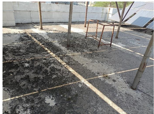
Sign of water clogging
