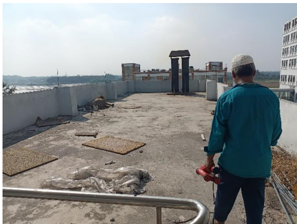
Insufficient discharge point
