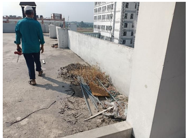
Sign of water clogging
