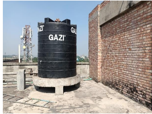
Plastic water tank on roof
