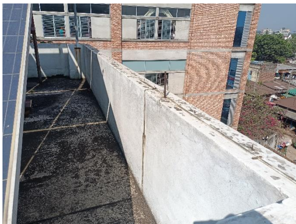
Insufficient discharge point
