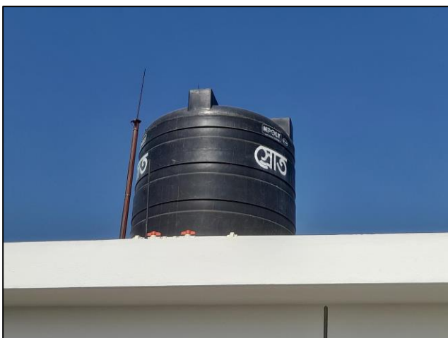
Unbraced PVC tank on the roof
