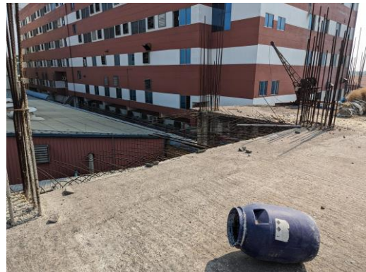
Falling Hazard on roof level
