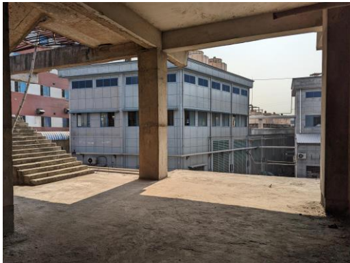
Falling Hazard on 1 st floor
