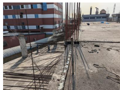
Corrosion in exposed rebars
