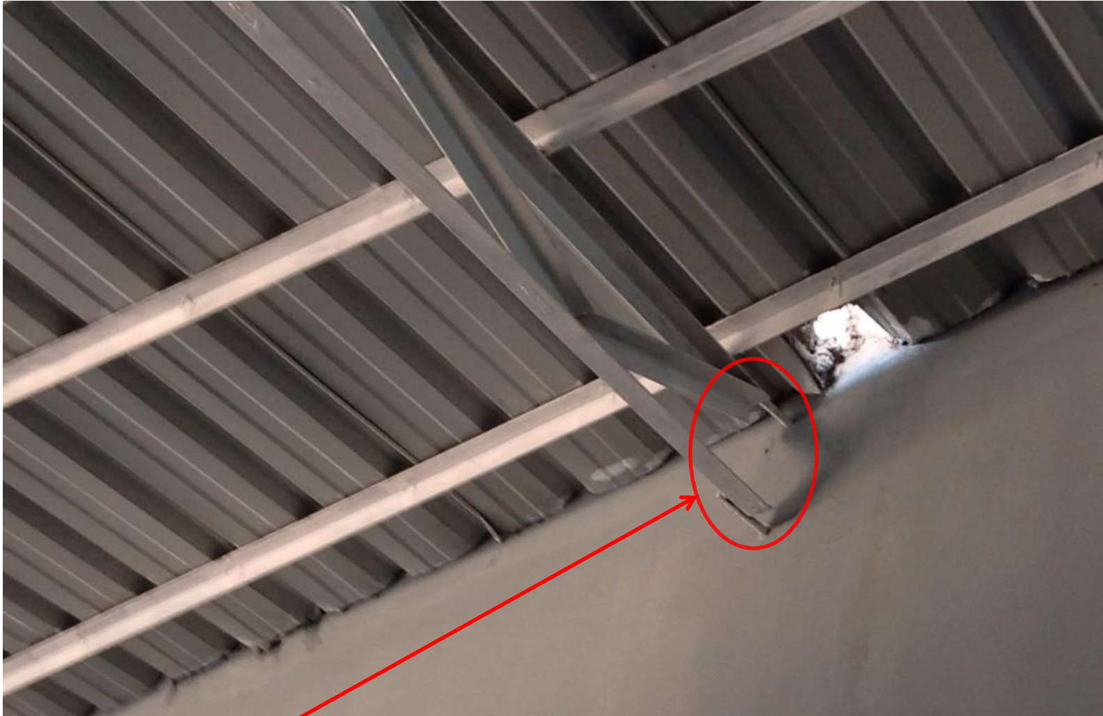
Non engineered truss supports
