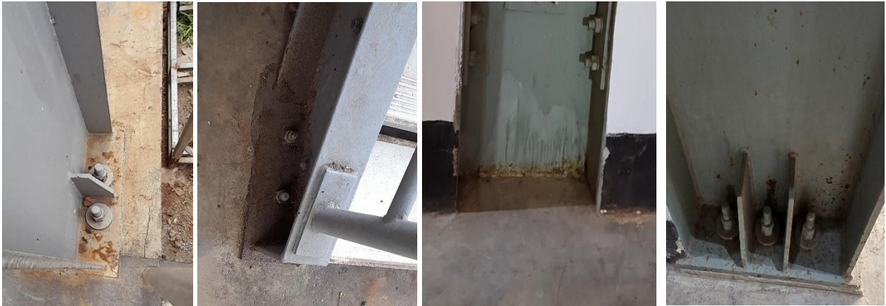
Image of corrosion
