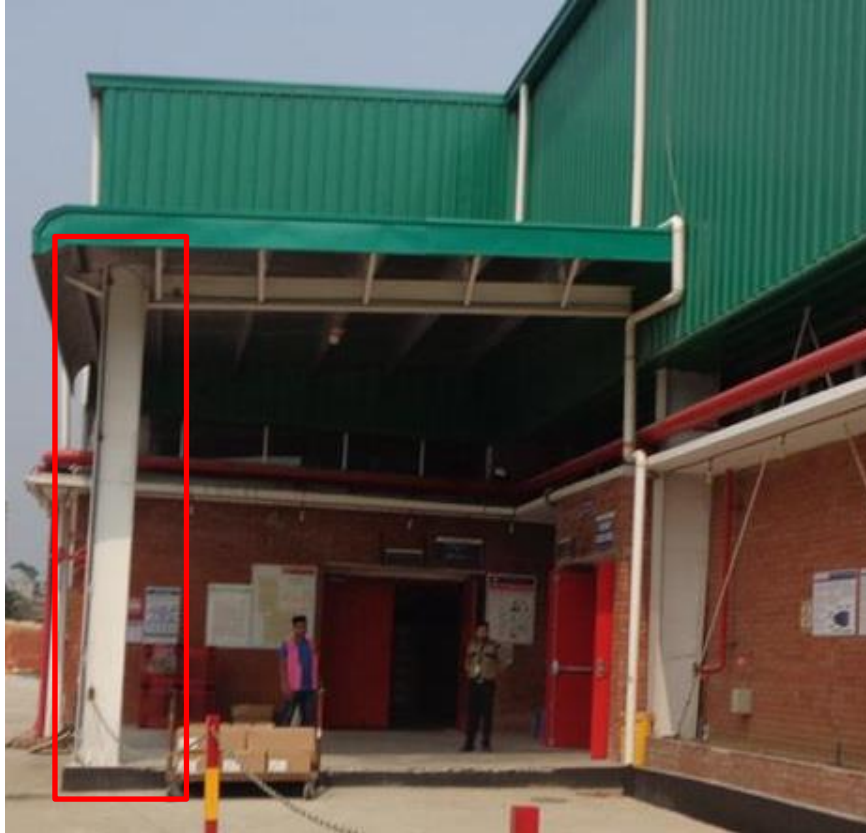
Steel Column susceptible to vehicle impact
