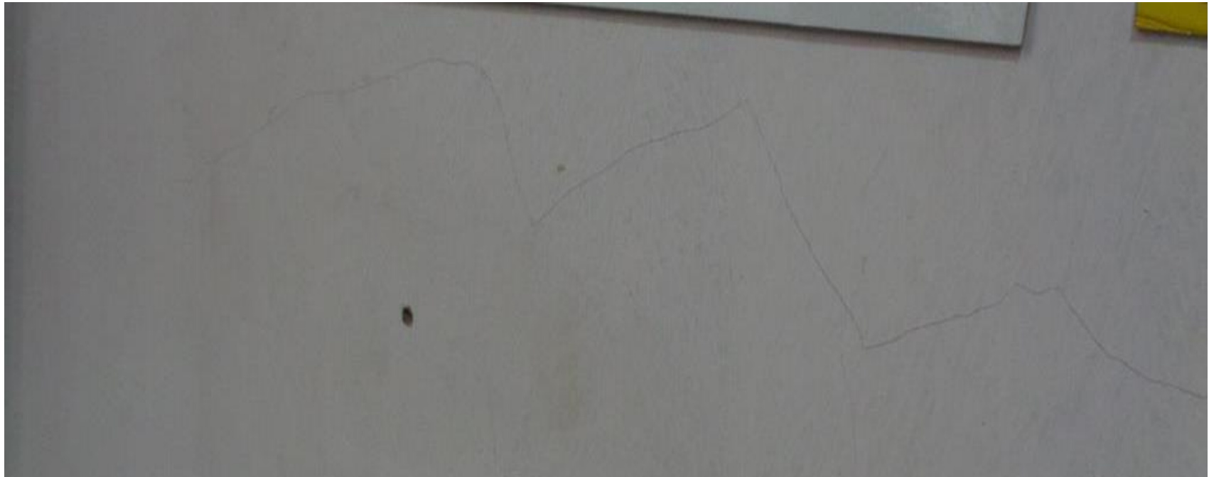
Cracks in retaining wall
