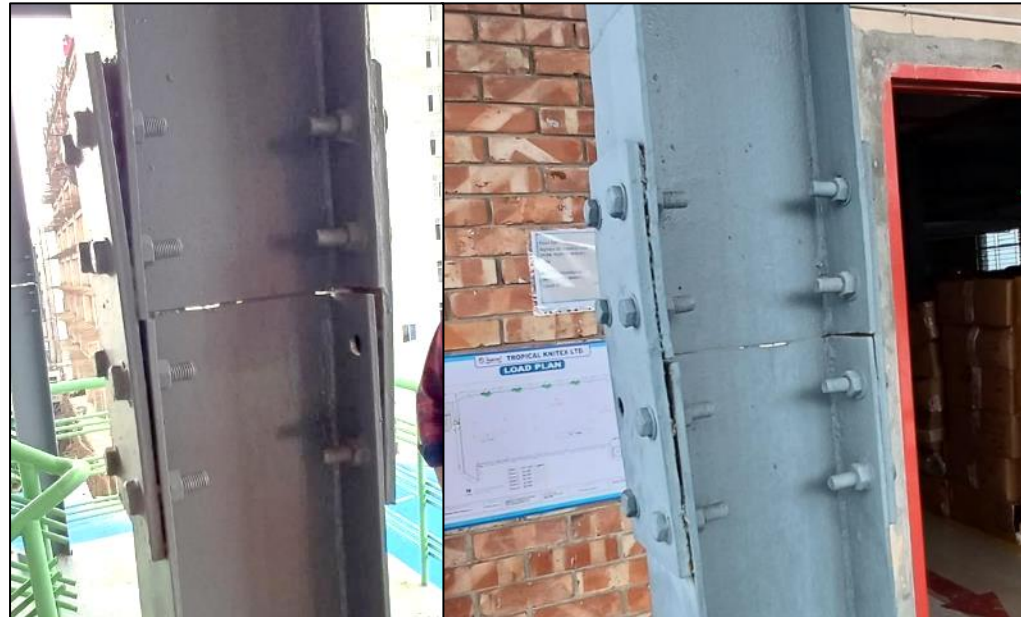
The poor connection found in steel stair-1
