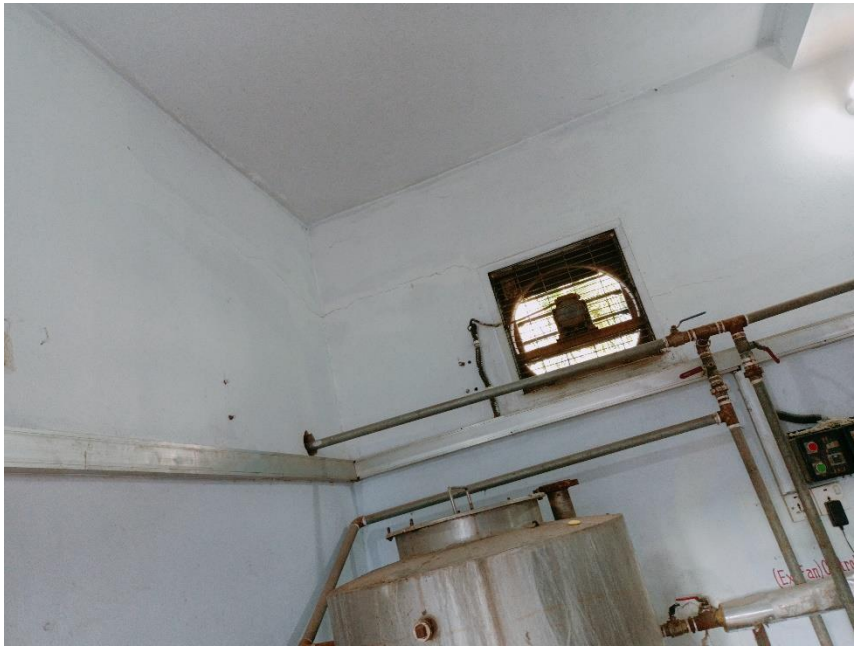
Compressor & Boiler Room
