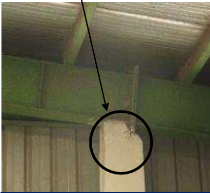
Column top broken at the joint of rafter at south end bay
