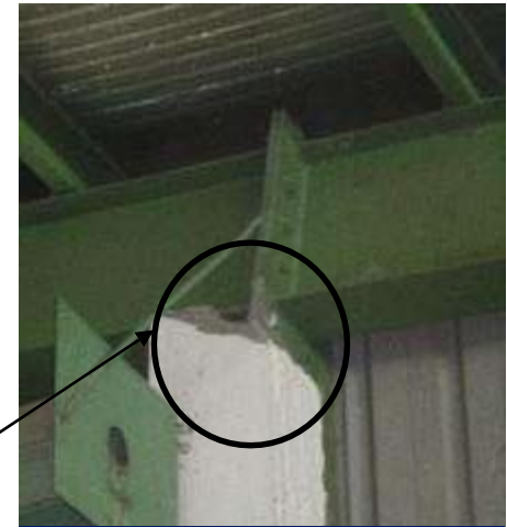
Column top broken at the joint of rafter at north end bay
