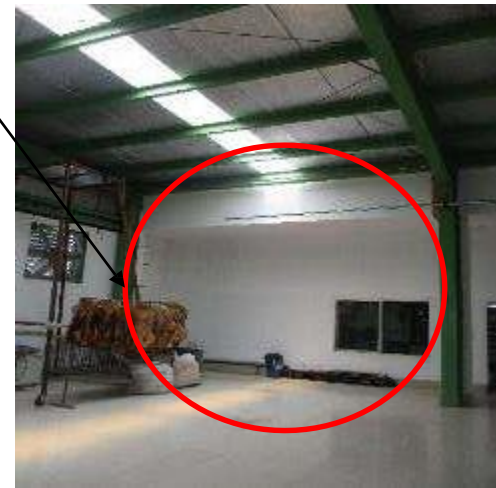
No vertical bracing was observed on east side
