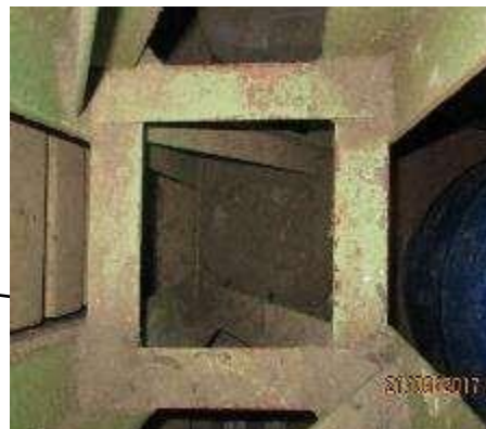
Cross section of steel column on site which is different than provided drawing
