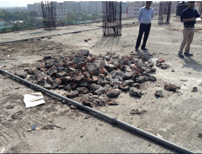
Uncontrolled storage materials
