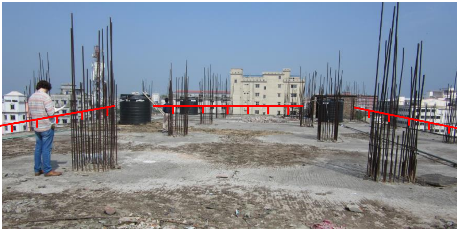
No edge protection on the roof
