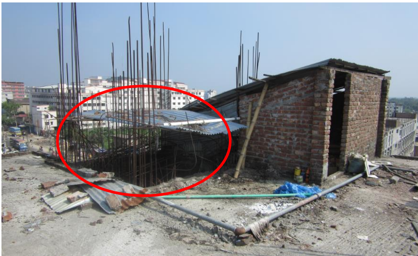
Unprotected lift shaft
