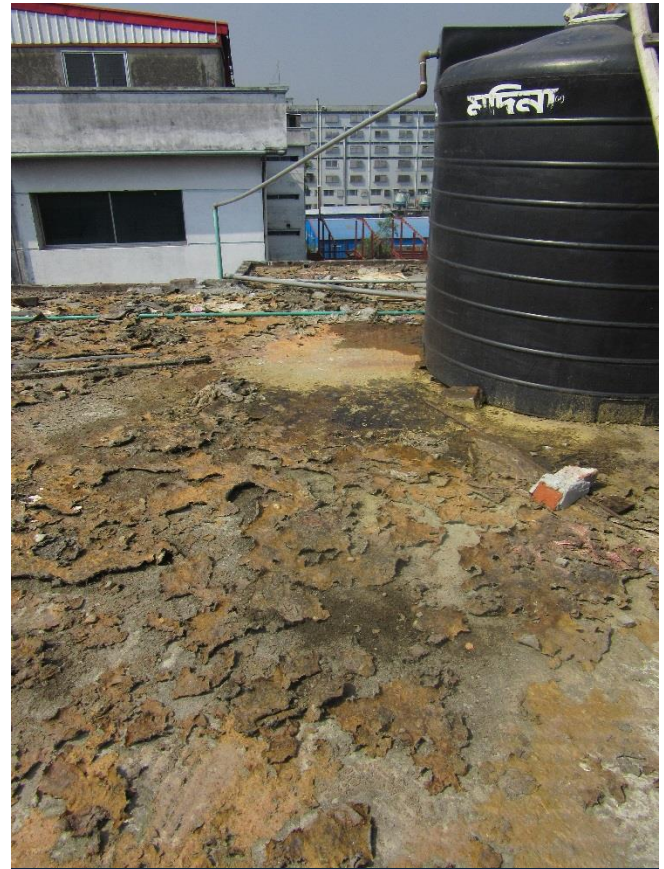
Roof slab degradation
