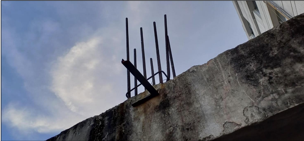
Exposed rebar of Column
